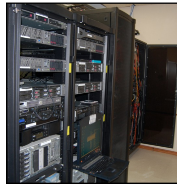
Network Server Room At City Hall
